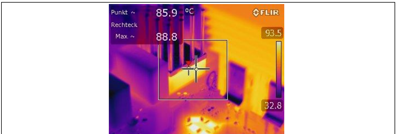
Figure 32 Thermal image of the input rectifier
