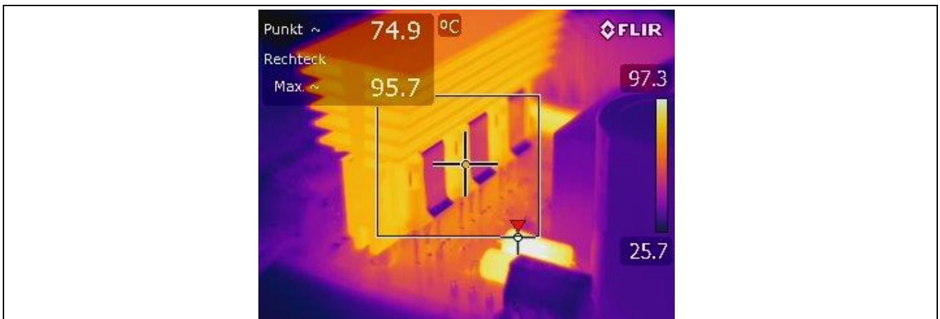
Figure 31 Thermal image of right power MOSFETs (hotspot at the capacitor's balancing resistors)
